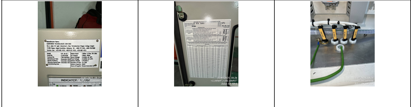
BATTERY CHARGER (COMPLETE WARRANTY STICKER) OVERVIEW OF BATTERY CHARGER (COMPLETE WITH 30VDC LOW MAINTENANCE SYSTEM COMMISSIONING CHECKLIST) INSIDE BATTERY CHARGER INDIVIDUAL EARTHING CONNECTIONS COMPLETED FOR I/O CABLES TO EARTH STUD AT RCB PANEL
