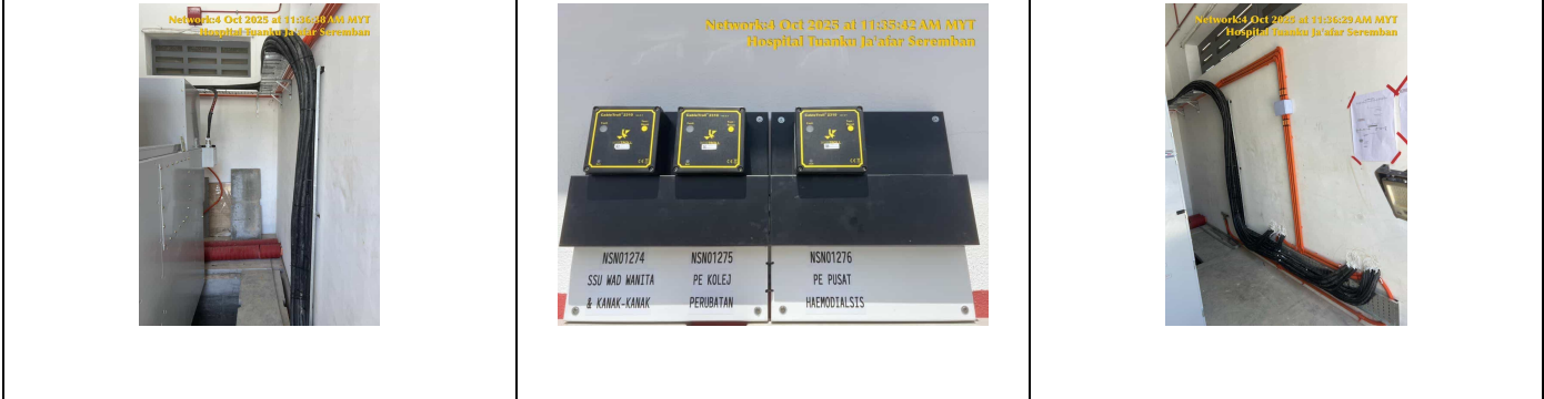
OVERVIEW OF EFI(S) AFTER INSTALLATION OVERVIEW OF EFI(S) AFTER INSTALLATION SECOND PICTURE (IF ANY) OVERVIEW OF EFI(S) AFTER INSTALLATION THIRD PICTURE (IF ANY)
