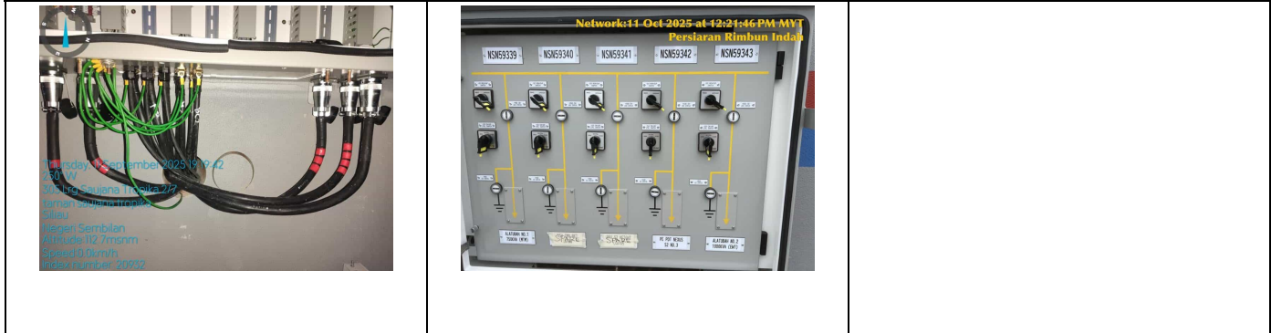
SAMPLE OF COMPLETED MULTI-CORE CABLE TERMINATION (INSIDE RCB) SECOND PICTURE (IF ANY) SAMPLE OVERVIEW OF RCB'S SINGLE LINE DIAGRAM (COMPLETE WITH FEEDER NUMBERS) SAMPLE OVERVIEW OF RCB'S SINGLE LINE DIAGRAM (COMPLETE WITH FEEDER NUMBERS) SECOND PICTURE (IF ANY)
