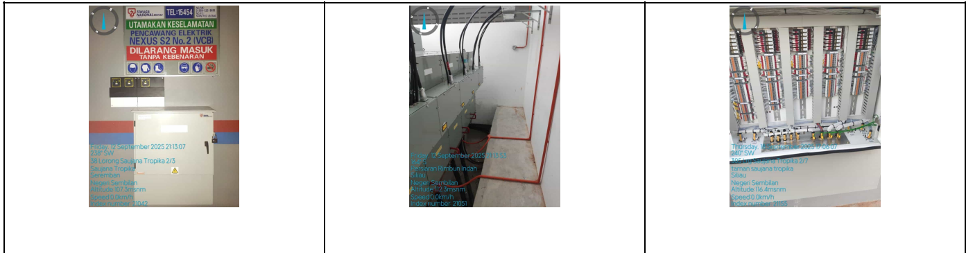
OVERALL PICTURE OF SUBSTATION OUTER WALL (WITH SUBSTATION NAME) SAMPLE OF COMPLETED MULTI-CORE CABLE TERMINATION (AT SWITCHGEAR'S SIDE) SAMPLE OF COMPLETED MULTI-CORE CABLE TERMINATION (INSIDE RCB)
