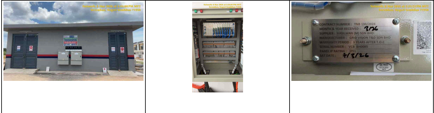
OVERALL PICTURE OF SUBSTATION OUTER WALL (WITH SUBSTATION NAME) RTU AFTER INSTALLATION (WITH INSIDE PICTURE) RTU WARRANTY STICKER (COMPLETE WITH SAT DATE)
